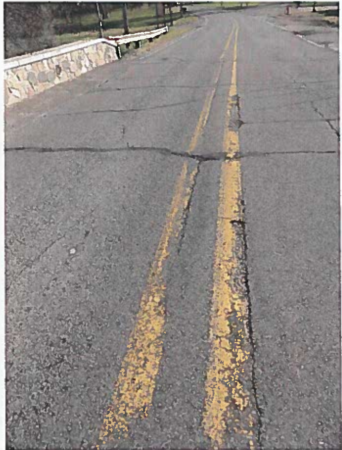
Document Name: 052.JPG Category: Deck Span Number: Comments: Cracking & spalling in bridge surface.
