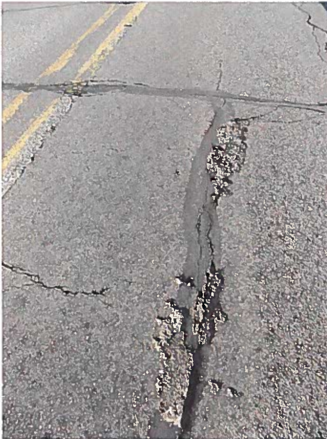
Document Name: 051.JPG Category: Deck Span Number: Comments: Typical surface cracking & spalling.
