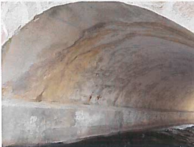
Document Name: 053.JPG Category: Other Span Number: Comments: Typical cracking and rust staining at arch repairs.
