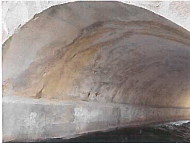
Document Name: 053.JPG Category: Other Span Number: Comments: Typical cracking and rust staining at arch repairs.
